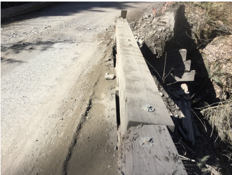
Downstream left bank guardrail condition
